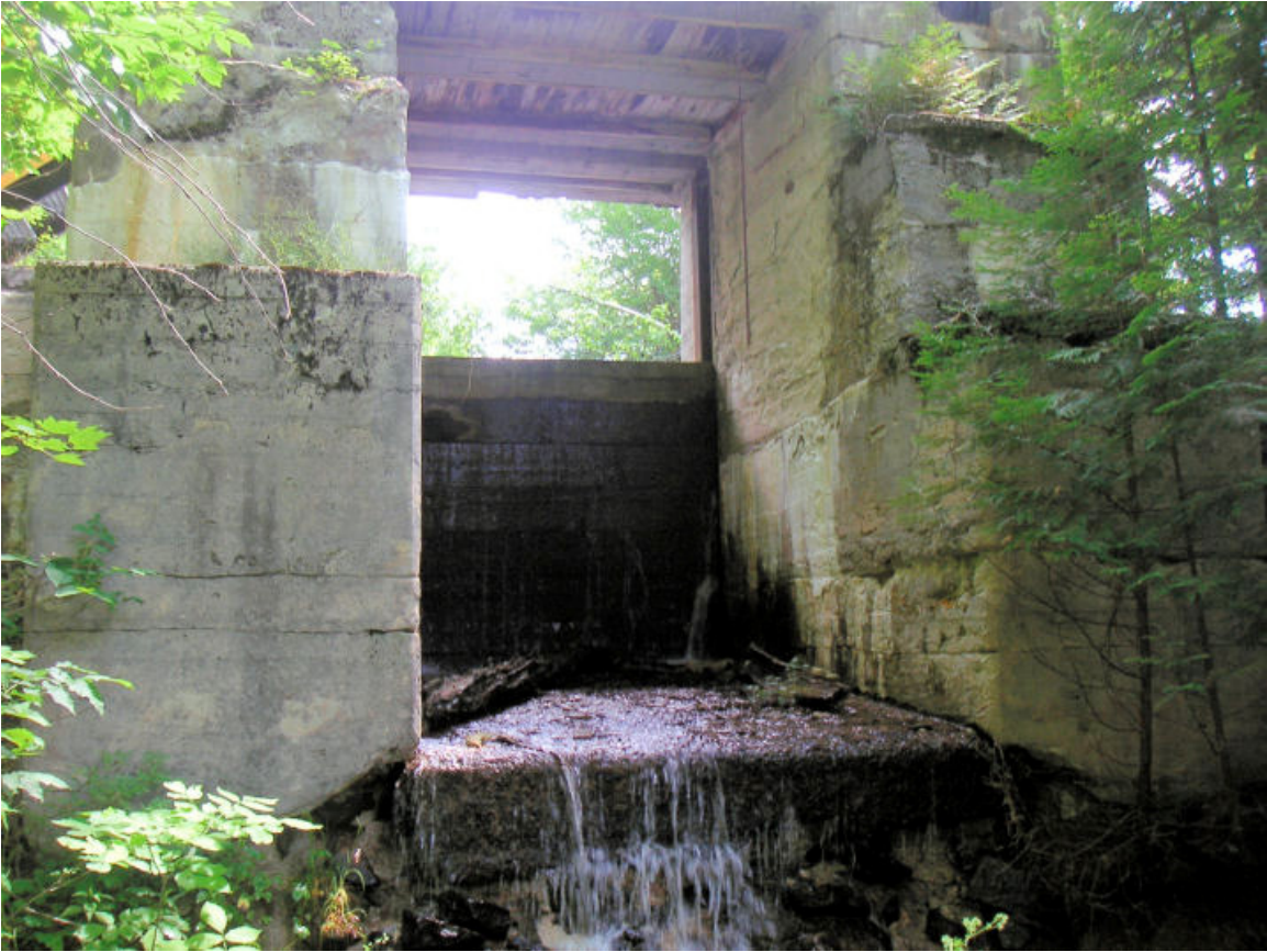
View from the bottom of the dam, with all (7) logs in place.
