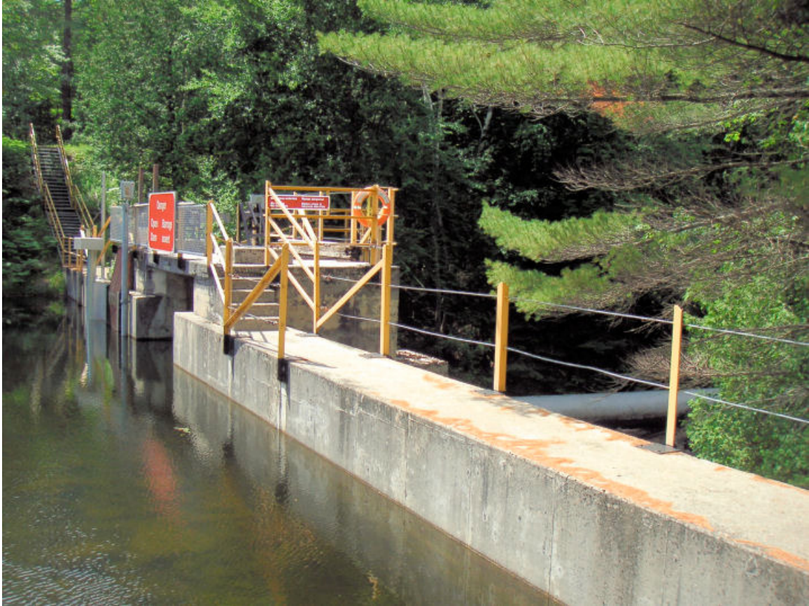
View from the top of the hydro dam (with water flow pipe seen to the right)
